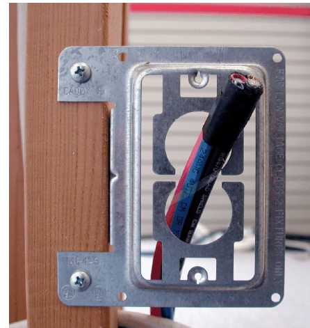
Mud Ring with Structured Cable. (Note that the cable needs yet to be secured.)
